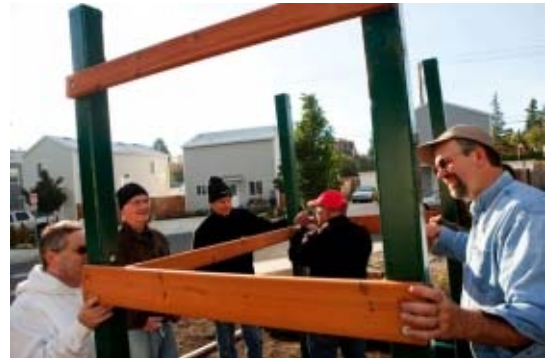
CHRISTOPHER ONSTOTT / BEAVERTON VALLEY TIMES Jim Valois, Norm Eder, Mark Forker and Craig Dirksen build a play structure for the children of nine low-income families in the Habitat for Humanity development at 160th and Farmington.
