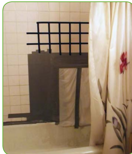
The Salazar bathroom walls are held together by duct tape and plastic
