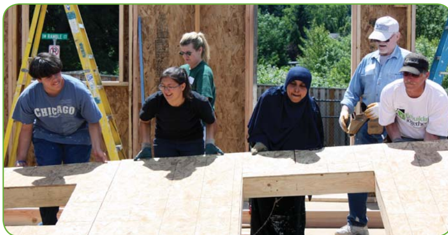
Volunteers work alongside family members and board president Dan Fako (in hat) raising a wall at Ramble Glen
